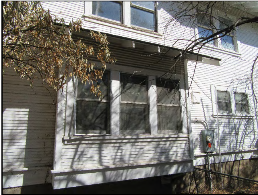
Boxed oriel windows with shed roof building, southern elevation (view toward north).
