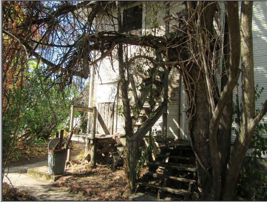
Figure 14. Rear entry to building, partially collapsed stairway, eastern elevation (view toward southwest), September 26, 2019.
