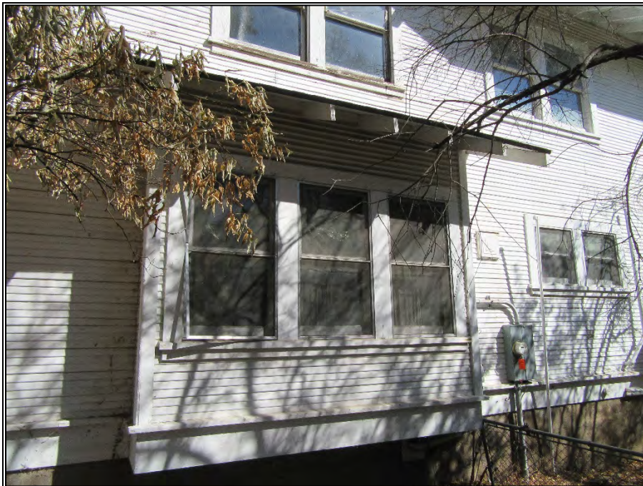
Figure 11. Boxed oriel windows with shed roof on the southern elevation (view toward north), September 26, 2019.
