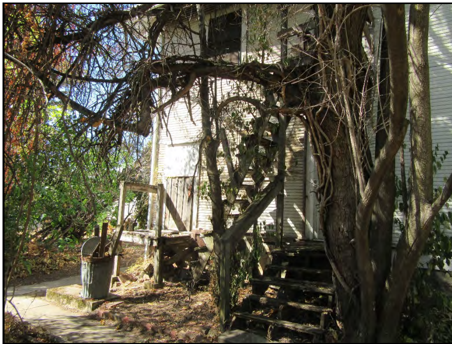
Rear entry to building, partially collapsed, eastern elevation (view toward southwest).
