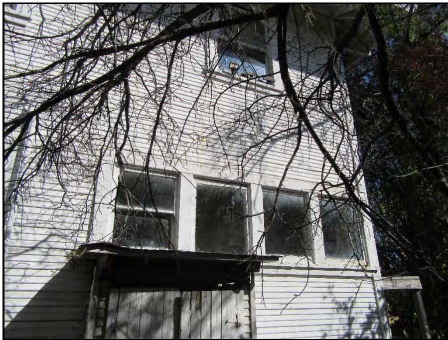
Wood framed, fixed and single hung windows, southern elevation (view toward north).
