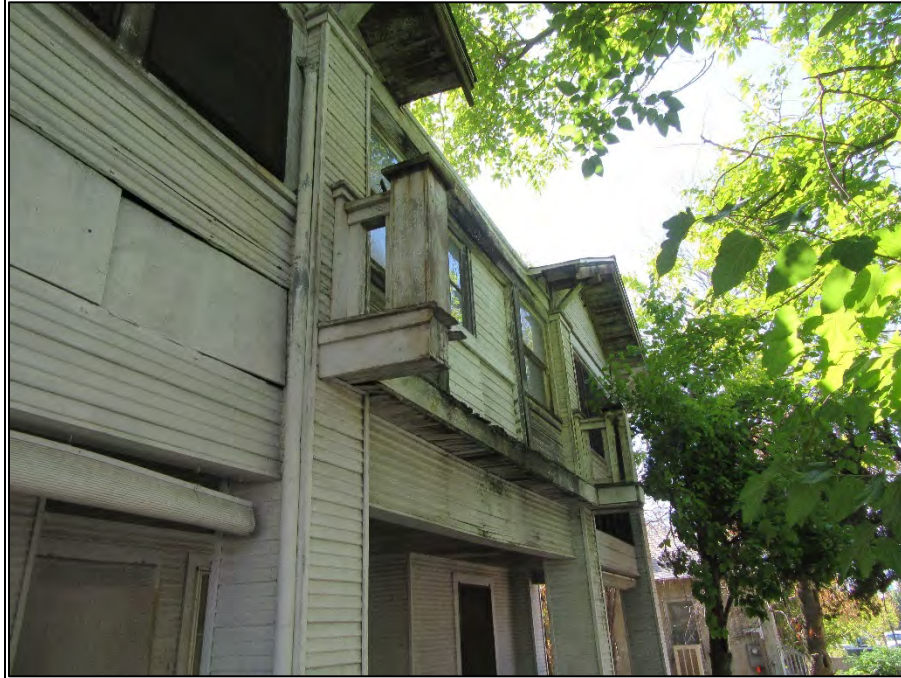
Figure 8. Second-story balcony has been removed, western elevation (view toward southeast), September 26, 2019.
