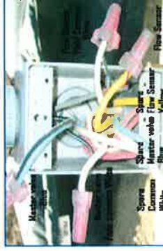
Master valve wiring installed correctly.
